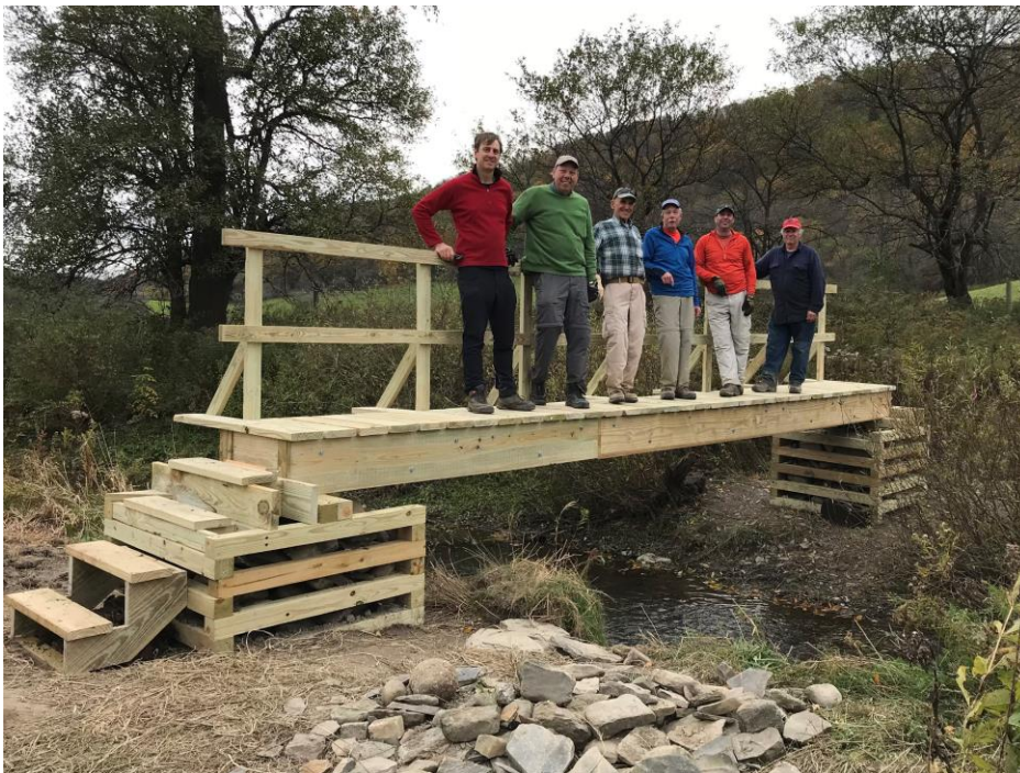
Bridge over Mud Creek built by the ADK-ON crew as part of the new trail construction connecting Cuyler Hill State Forest to Mariposa State Forest which eliminated a 4 mile road walk. Pictured: Harold Kyle, Dave Grant, Ken Kaufman, Dick Harper, Bob Rosati, Mike Ogden. Photo Courtesy Dick Frio
