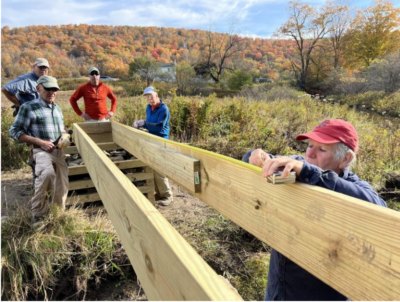
Dave Grant, Ken Kaufman (Project Engineer), Bob Rosati, Dick Harper, Mike Ogden (Project Construction Manager) building the bridge to span Mud Creek on the new trail, Photo Courtesy Harold Kyle
