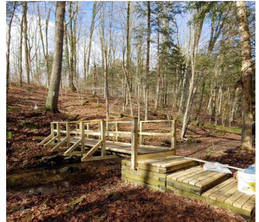
Bridge built by the ADK Onondaga crew in Mariposa State Forest last year.
